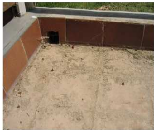
Evidence of stagnant water
