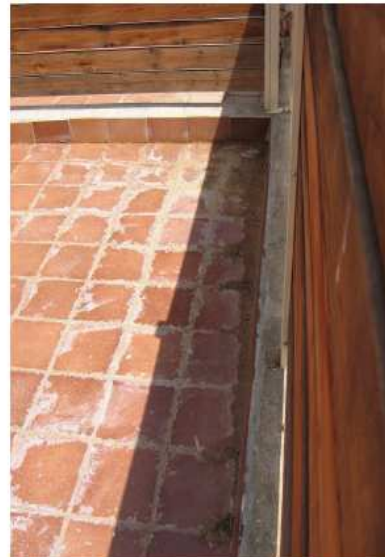
Saltpetre at the joints
